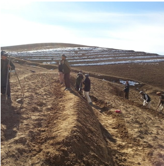
Establishment works on the terraces in Sari Joy village (Mia Jan Maroofi)
