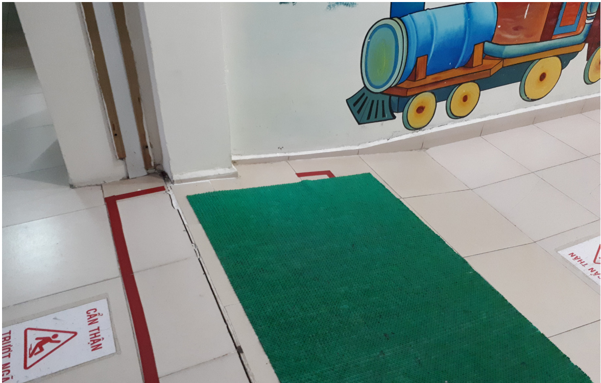
Figure 32: The floor on the right and on the left were on the same level when this hospital in Long Xuyen was built
