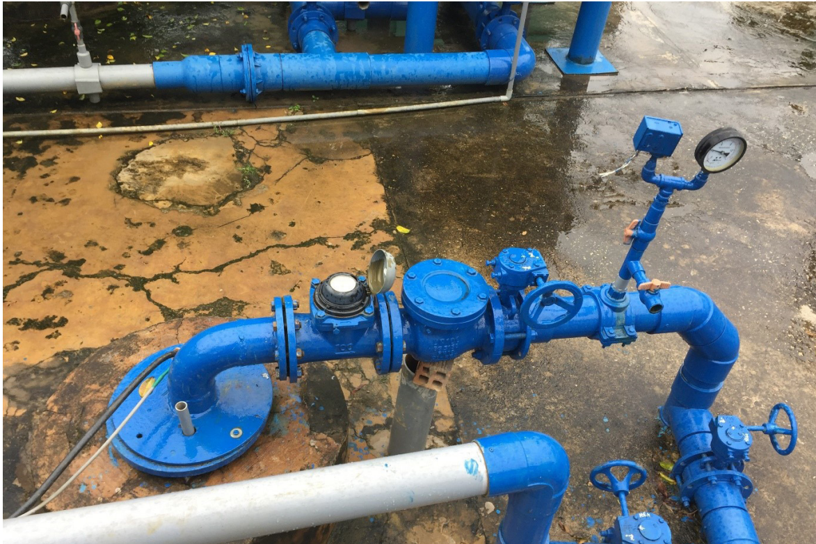
Figure 37: Groundwater pump connection for commercial drinking water supply in Ca Mau (Photo credit: BGR)
