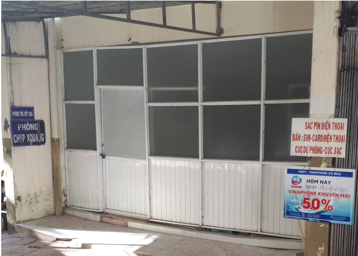
Figure 31: The centre of the ground floor is sinking faster than the walls, resulting in gaps between the window divider, the door, and the floor (a hospital in Ca Mau).
