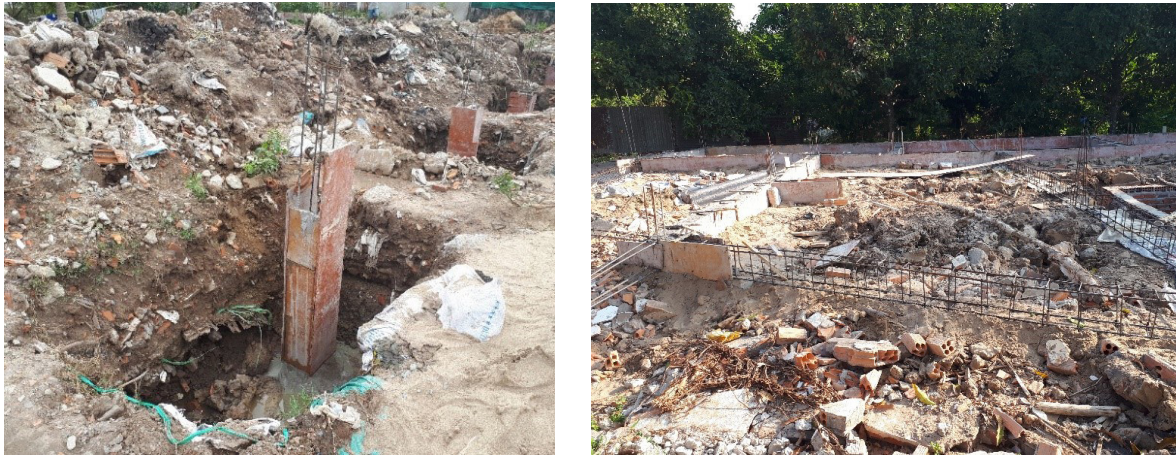
Figure 21: Left: Foundation of a pillar of a residential building in Can Tho. Depth approx. 1 m. Right: The walls have no foundation at all.
