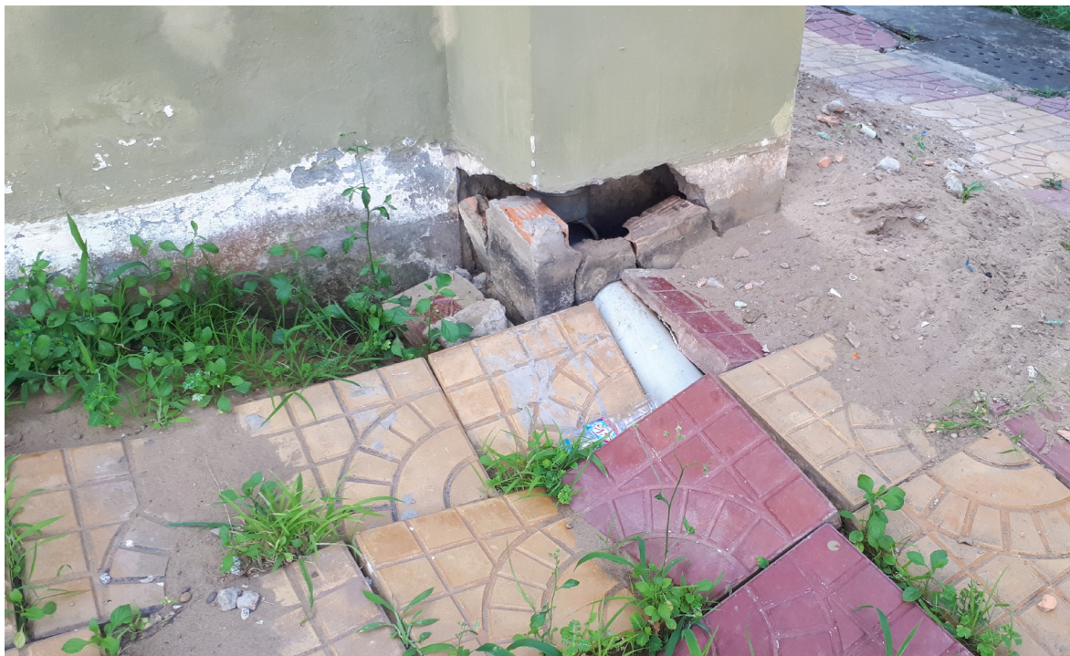
Figure 30: Disconnected rain drainage pipe (hospital in Ca Mau). The structure of buildings may be compromised by land subsidence.
