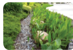
Filter drains or gravel trenches
