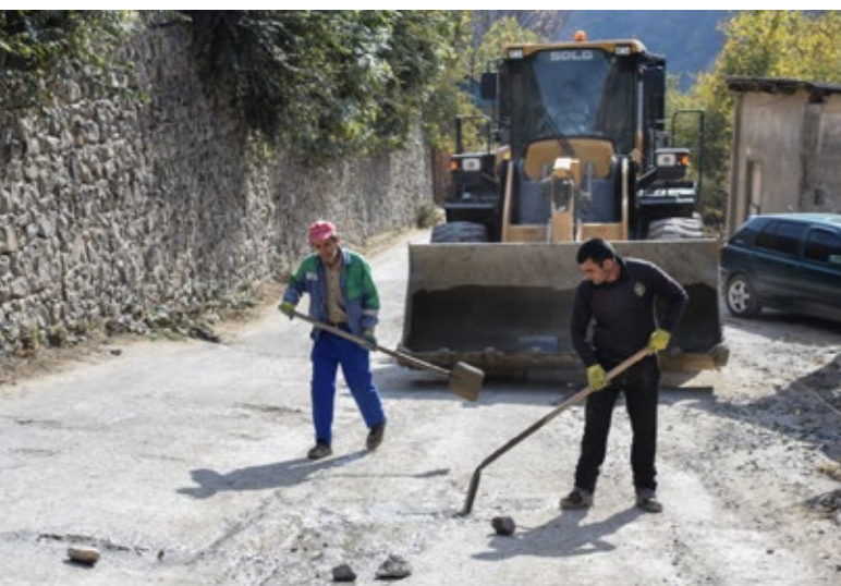
Following the consolidation of municipalities in Armenia, a series of construction works were implemented in the municipality of Akhtala. ©GIZ
