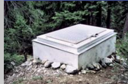
Vault containing measuring equipment
