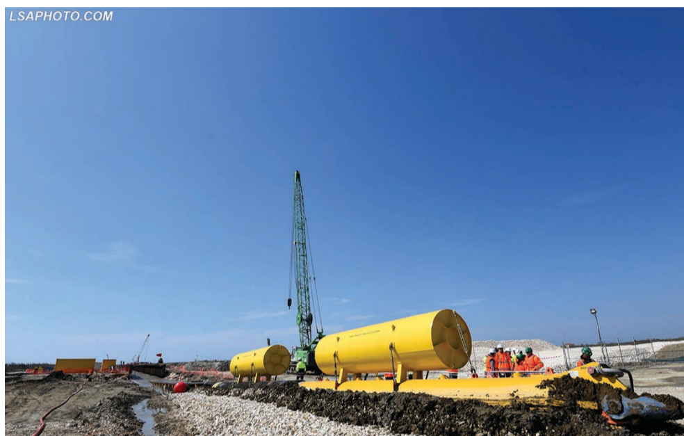
Trans Adriatic Pipeline
