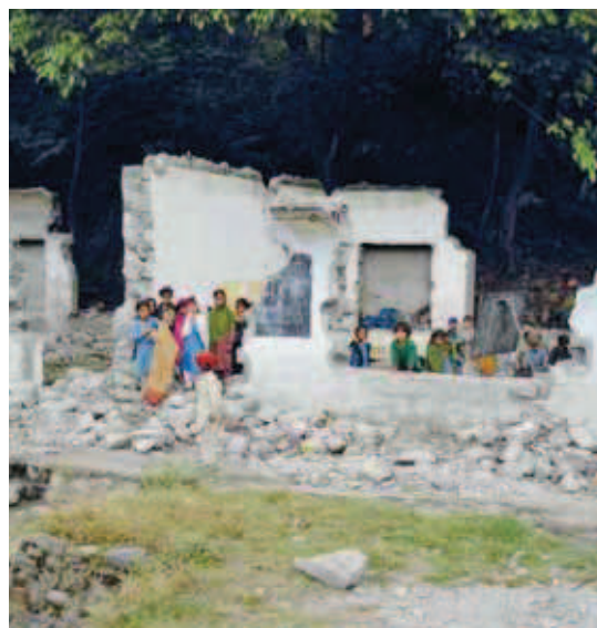
School building demolished by the October 2005 earthquake. Location: Chham, Muzaffarabad District, Azad Jammu Kashmir, Pakistan Photo credit: M.Zimmermann
