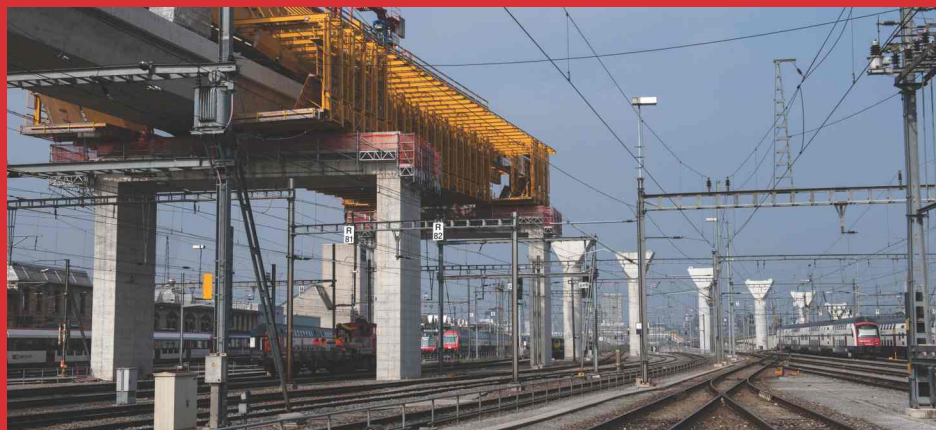
Construction of the new city cross link in Zurich, Switzerland (Photo: SBB AG)
