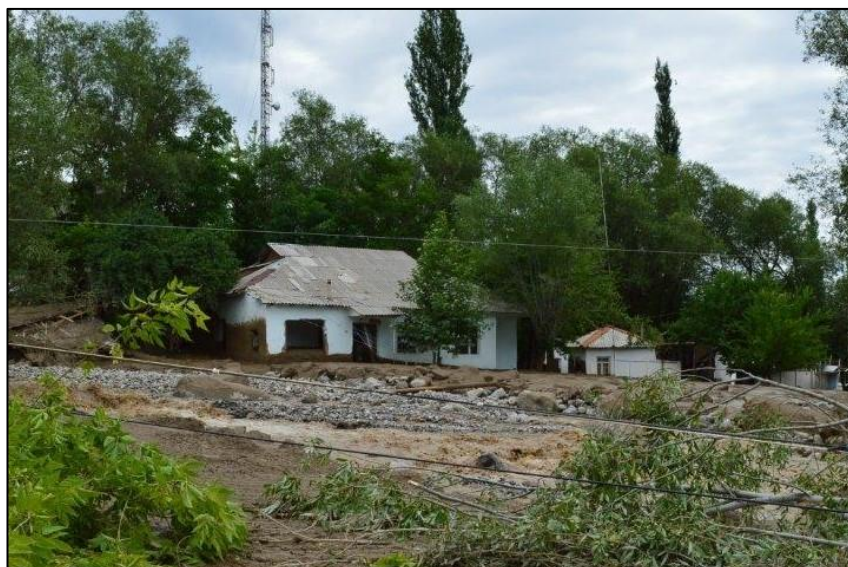
Damaged house in Gharm village of Rasht district. 4 July 2017. Photo credit: UNDP
