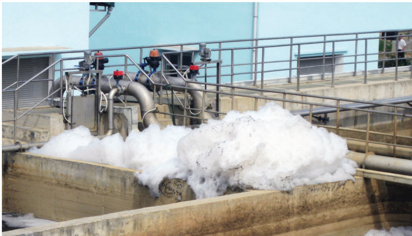
Vinh Wastewater Treatment Plant, Nghe An Province
