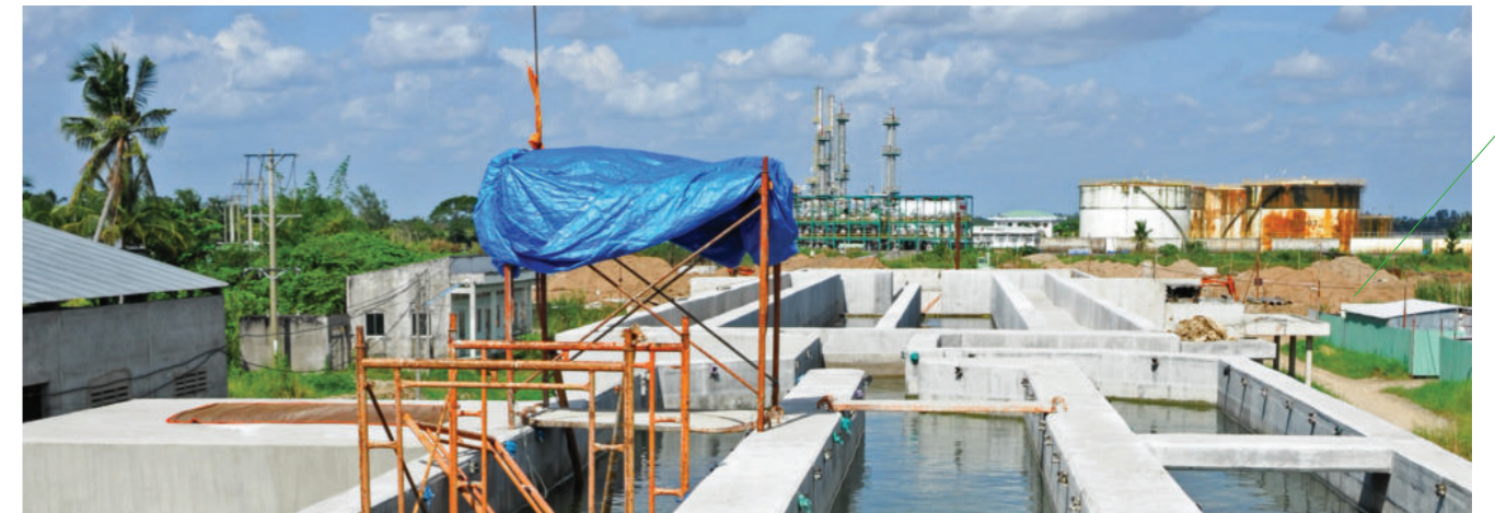
Soc Trang Wastewater Treatment Plant, Soc Trang Province
