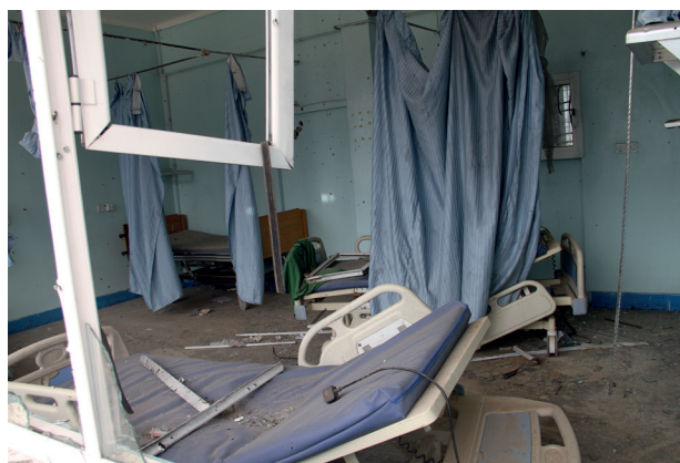
Yemen, Taiz city, Al-Thawra hospital. The three patients who had been laying in this room were pulled out of their beds when the shelling started. / Photo: AL ABSI, Wael
