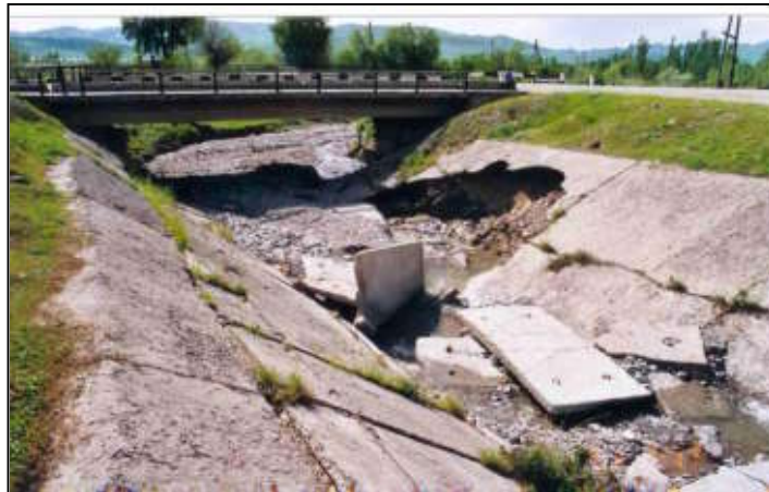
Figure 7: Lacking maintenance of riverbank protection structures can even increase the risk (Muminabad, southern Tajikistan)
